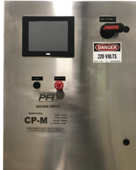
PLC CONTROLLER WITH TOUCH SCREEN INTERFACE ALLOWING EASY ACCESS TO STORED SETTINGS
